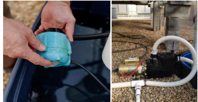
Figure 5. Two kinds of irrigation pumps that are used to move nutrient solution to plant channels. (Chris Mullins, Virginia Cooperative Extension)
