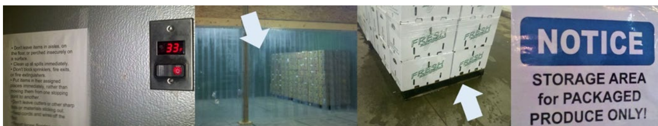
Figure 9. Produce storage from left to right: digital temperature display and posted rules on the outside door of a cooler; plastic vinyl curtain (arrow) at the entry of a large cooler area; packed vented produce stacked off the ground on a plastic pallet; and signage posted on outside of small walk-in cooler door. (Amber Vallotton, Virginia Cooperative Extension)
